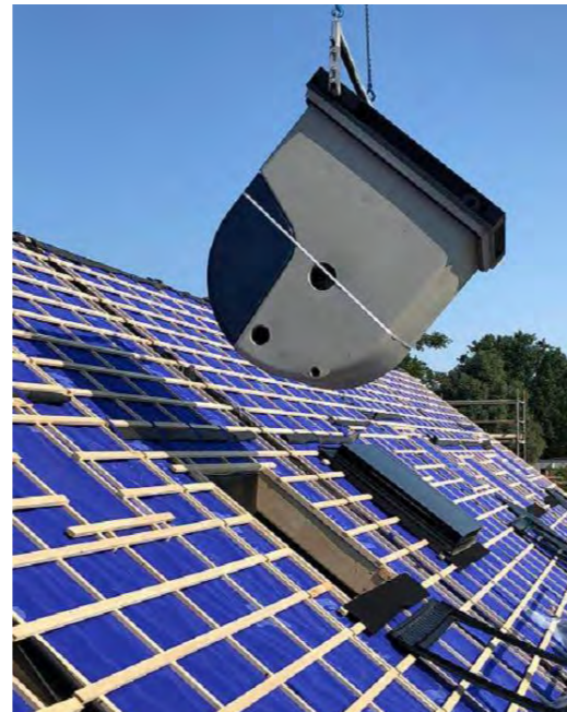
WTW installatie 'in daks'
